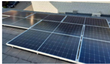
Project: Residential PV Power System in Germany Location: Germany Capacity: 7KW Grid Connection Time: 2023
