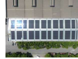
Project: Sunlit Factory Rooftop PV Power System in Wuxi Location: Jiangsu, China Capacity: 0.3MW Grid Connection Time: 2023
