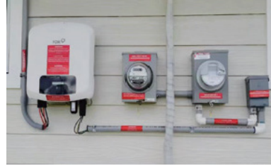
Project: Residential PV Power System in Palau I II Location: Palau Capacity: 2MW Grid Connection Time: 2022/2023
