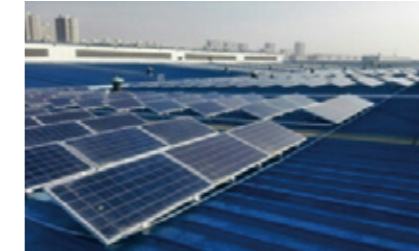
1.4MW KIPOR Rooftop PV Project
