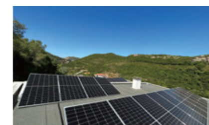
Clinic PV Power System in Portugal
