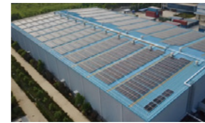
1.04MW Wuxi LONGI Materia Rooftop PV Project
