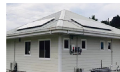
Residential PV Power System in Palau
